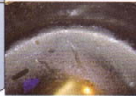
Picture of the tank's contaminated interior
